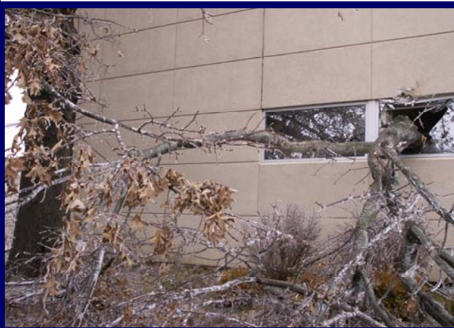
Above: Tree limb falls through window of City Attorney's Office at City Administration Building. Photograph by Rose Lawrence.
